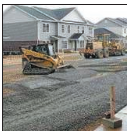
Construction workers prepare to pave the parking lots on Ridgcrest Town Apartments site.
